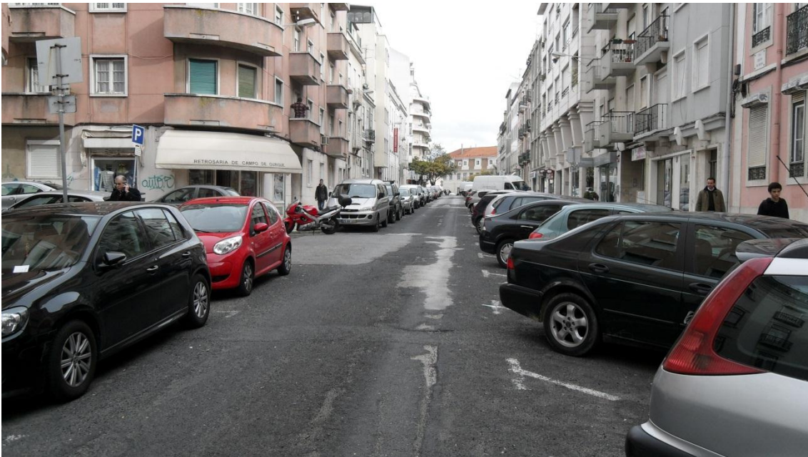
Figure 13 – Picture of pavement condition (before intervention).
