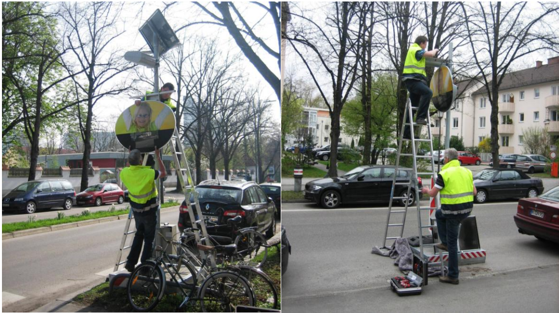
Figure 7 Installation of Dialog-Displays on Denningerstraße in Munich (Left direction Richard-Strauß-Straße; Spot 3; Right: direction: Herkomerplatz, Spot 1)
