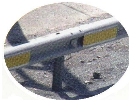
Illustration 22: Example of the linear delineation system 3M LDS Series 346 installed on a crash barrier.
