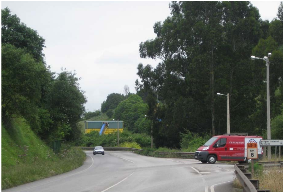
Illustration 14: In this photo it can be seen the conditions of the road marking before the campaign.
