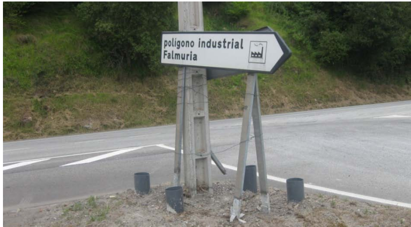
Illustration 29: The foundations for the new traffic signs and for the panels have been prepared.
