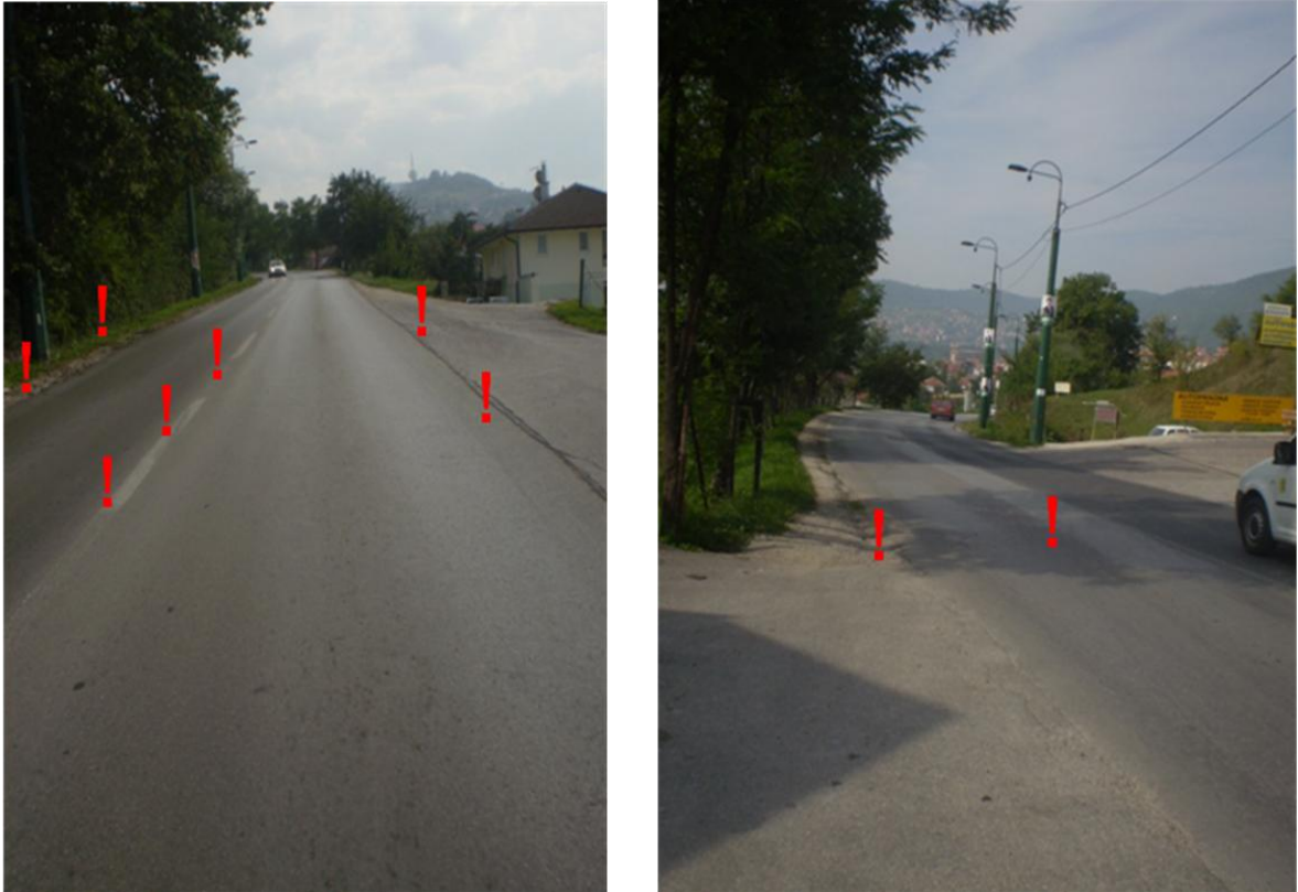
Picture 4: Problem: Lack of adequate road markings
