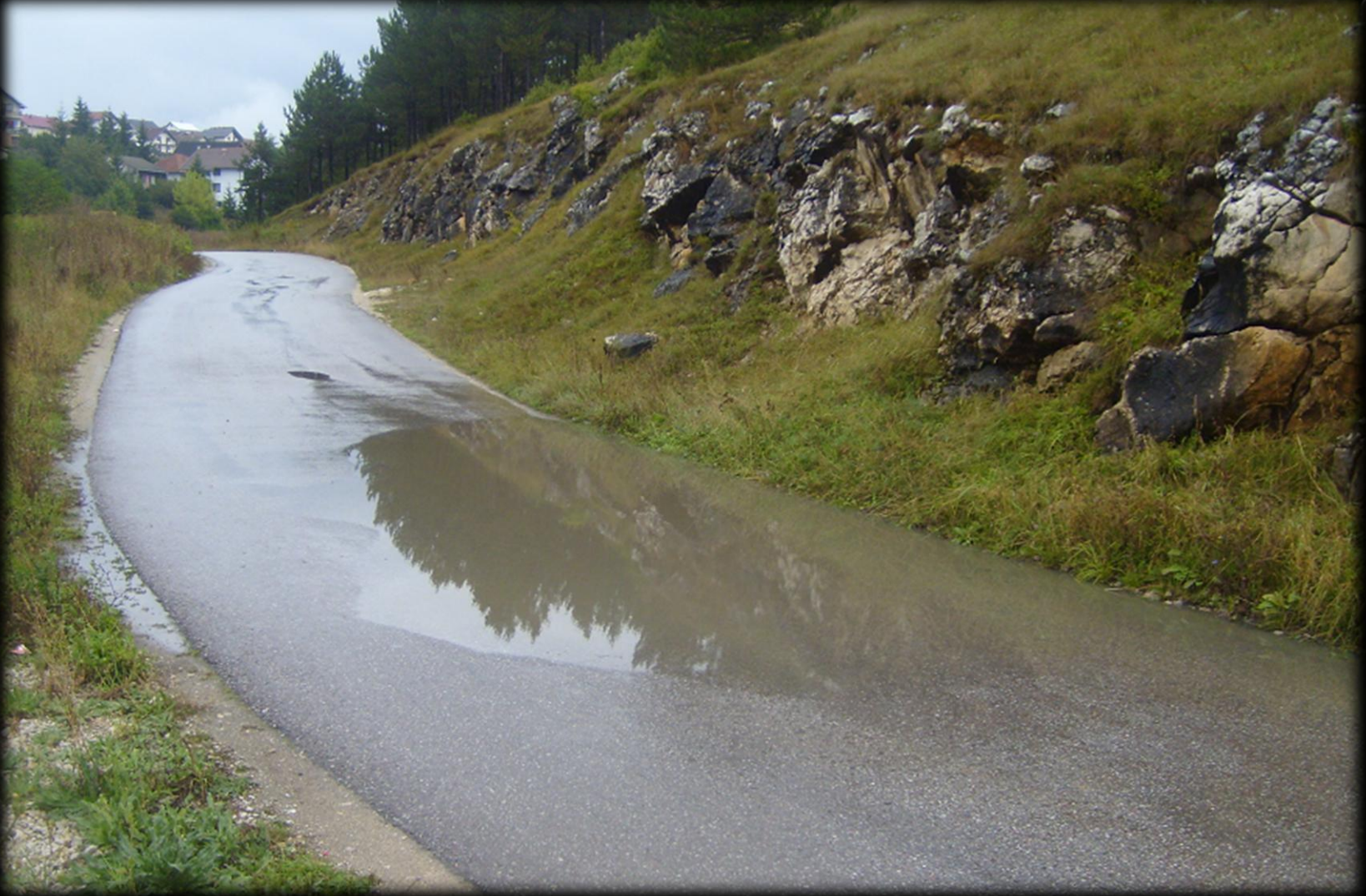
Figure 9. Frozen water in the winter makes safety situation worse
