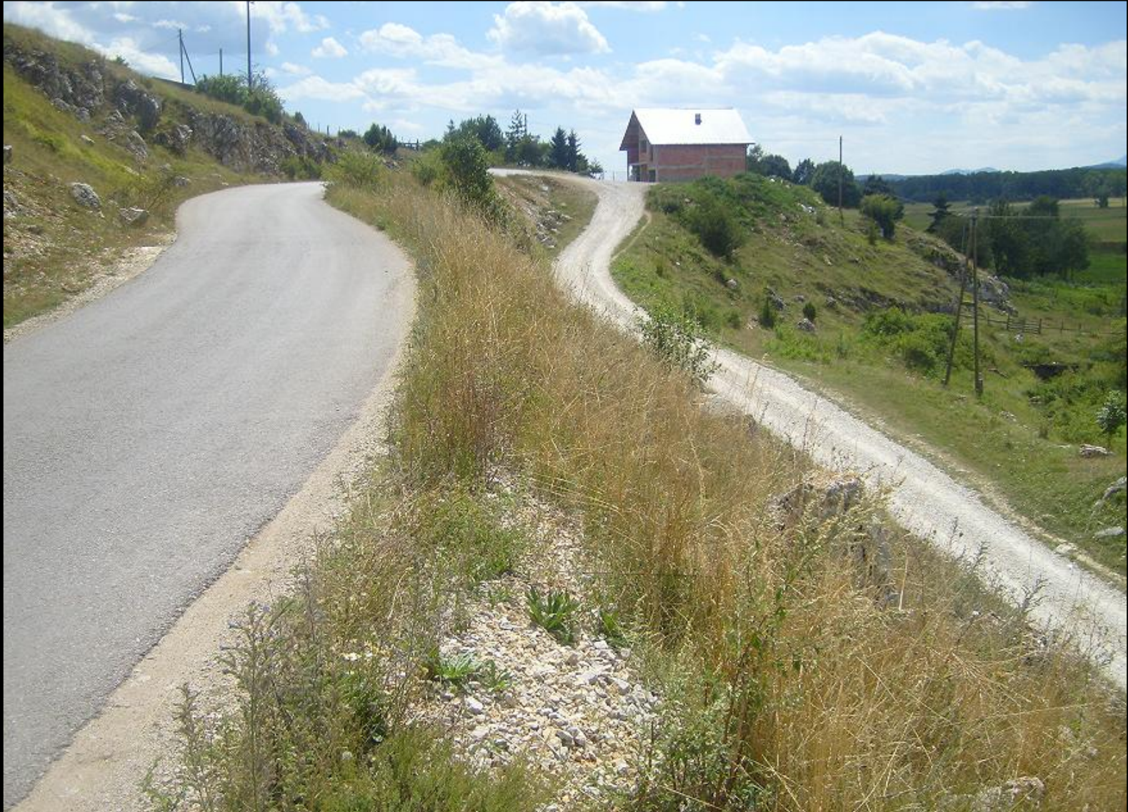
Figure 11. There is no protective crash barriers for vehicles
